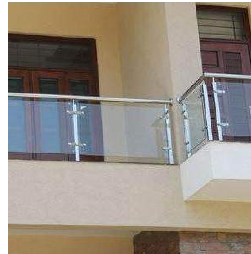
10- Aluminum and Glass Railing
